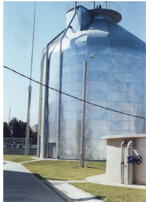
Figure 3. Anaerobic digester tank V = 1.500 \text{ m}^3 - Mangalia wastewater treatment plant.
